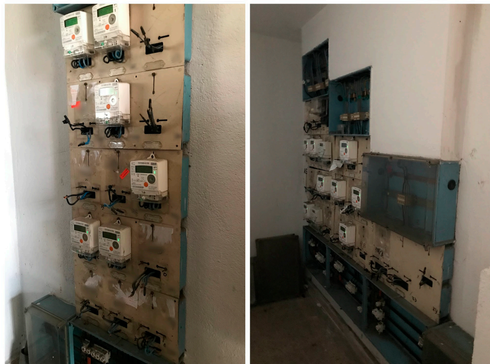
Figure 3. Power switchboard of the building located in the common area of the ground floor.
