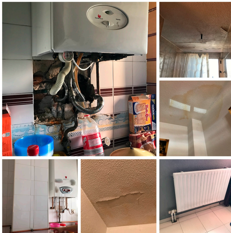
Figure 6. Images from the interior of the dwellings showing evident signs of dampness on ceilings and walls, as well as irregular and unsafe connections in gas boilers. The presence of heating emitters (radiators) does not result in their use by households due to other factors.
